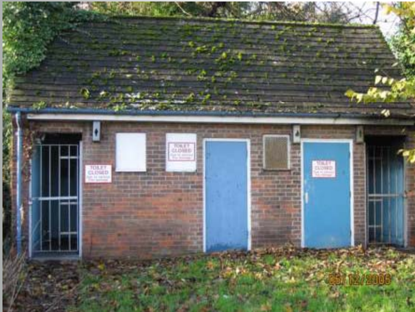
2005 Closed & Fire Damaged
