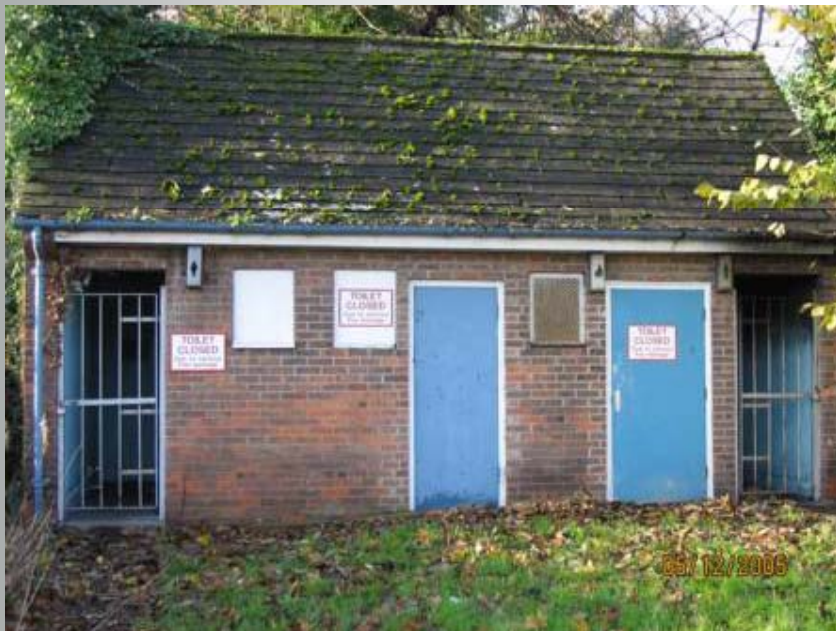
2005 Closed & Fire Damaged
